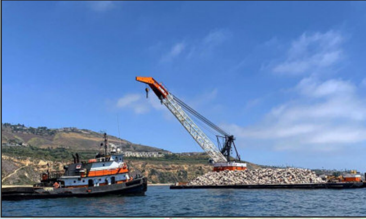
The construction crane and barge shot from the first day of construction on May 8. photo by Chelsea Williams
